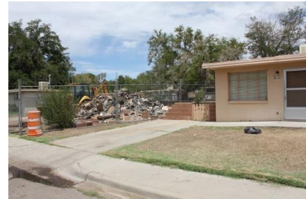
Photo of demolished residence.
