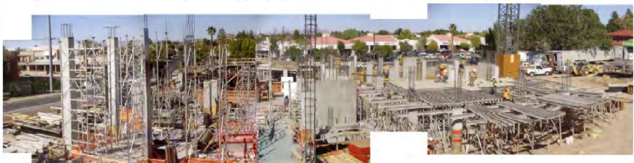
Shoring for Level 2 above Scene Shop & Shoring going up for Rehearsal Room – view from Conroy 2 nd Floor
